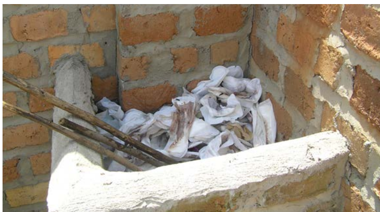
Image 4.8: Sanitary pads disposal point in a latrine block. The pads dry out before being burnt.
