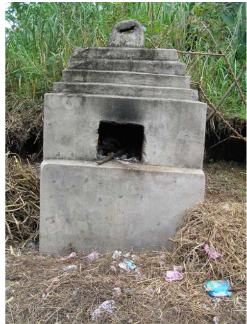
Image 4.7: Incinerator without a door
