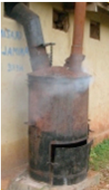
Image 4.9: A high-temperature incinerator, capable of burning sanitary pads
